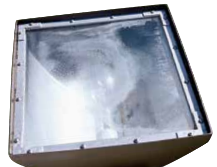
Figure: Luminaire with condensation
